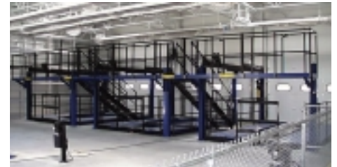
Lube Racks — Mezzanine, 3 bay
